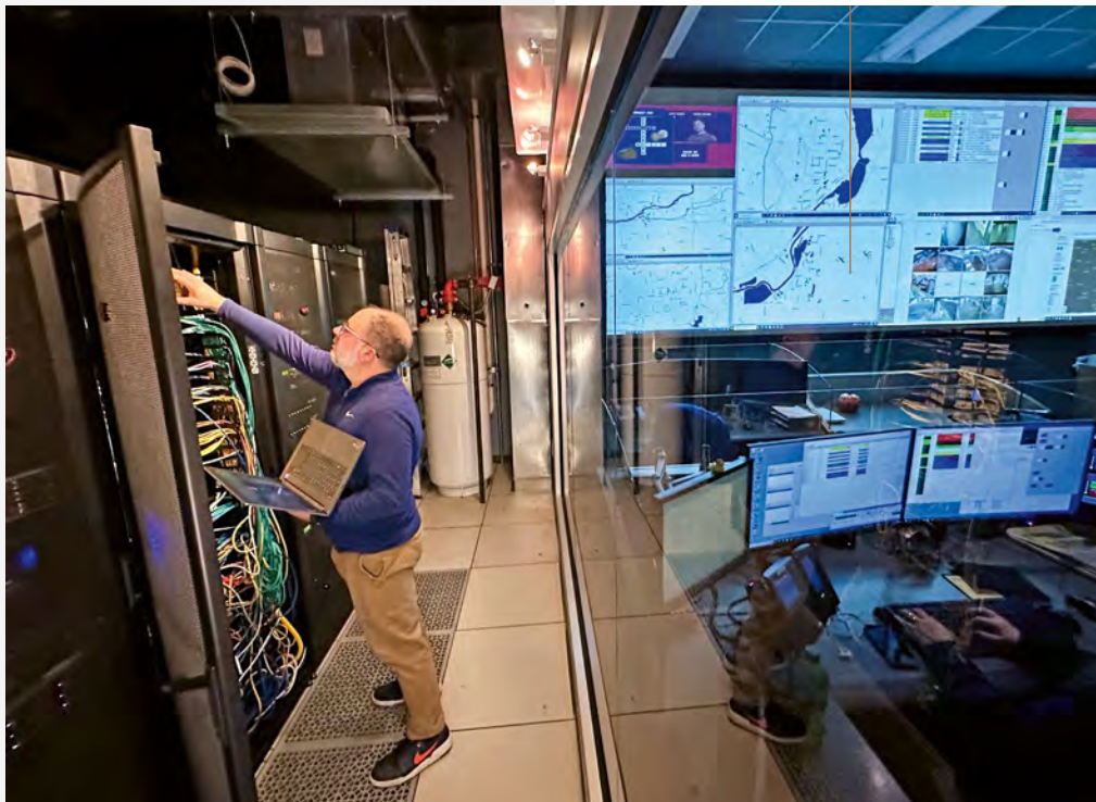
McGee conducting systems maintenance in the data center adjacent to AMT's dispatch center
